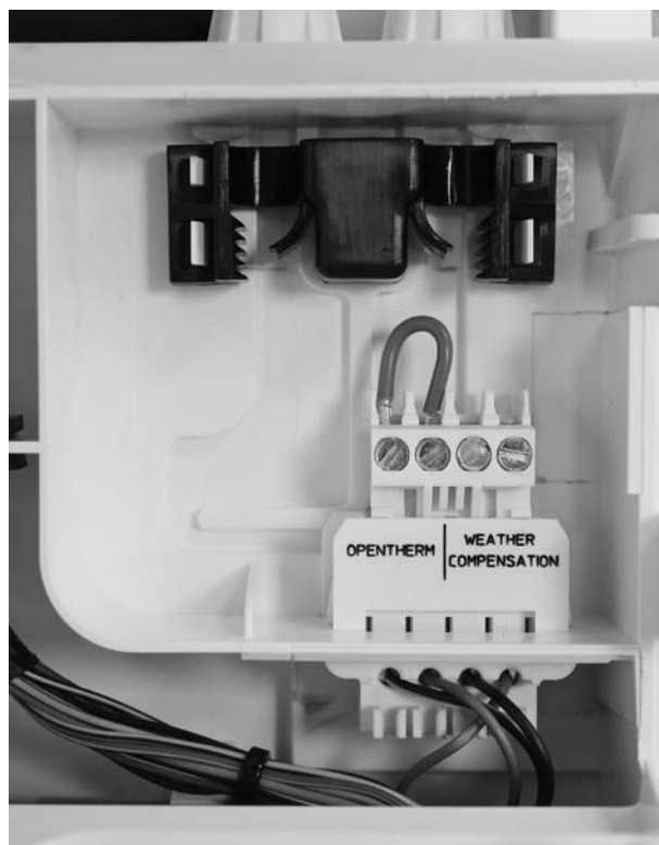
INSTALLER CONNECTIONS (RHS)
