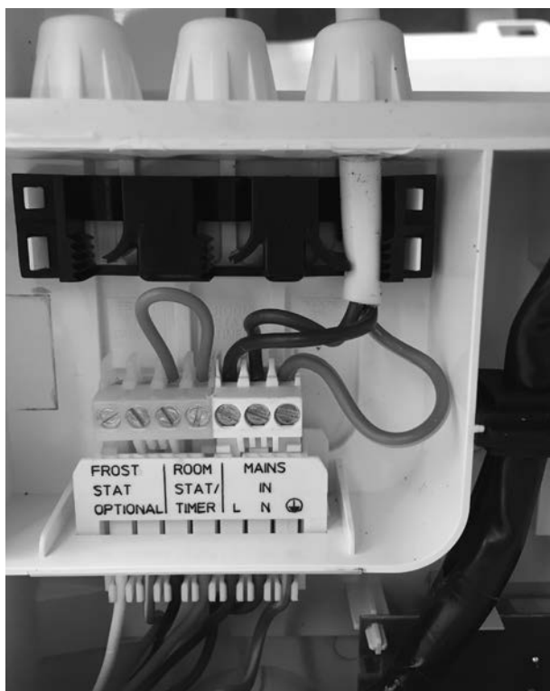
INSTALLER CONNECTIONS (LHS)
