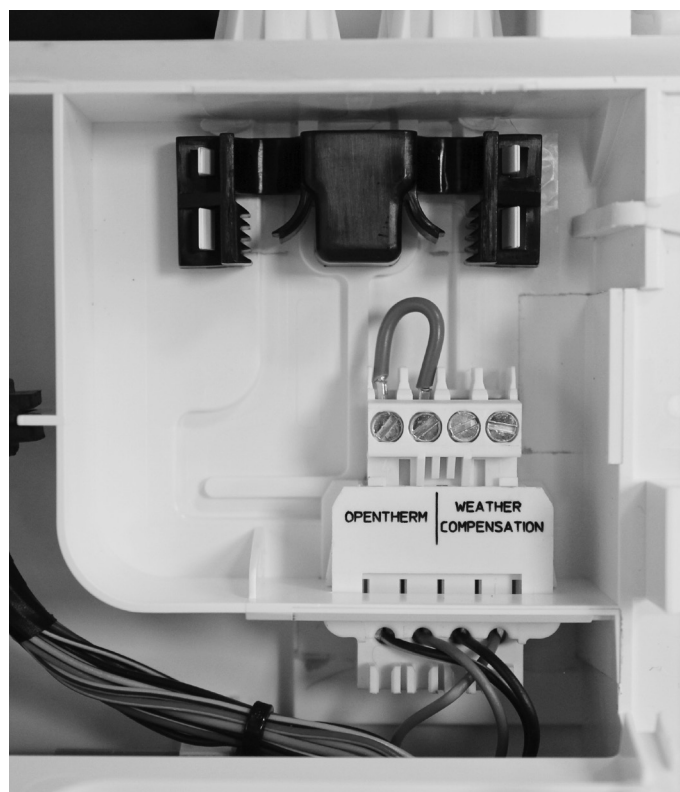
INSTALLER CONNECTIONS (RHS)
